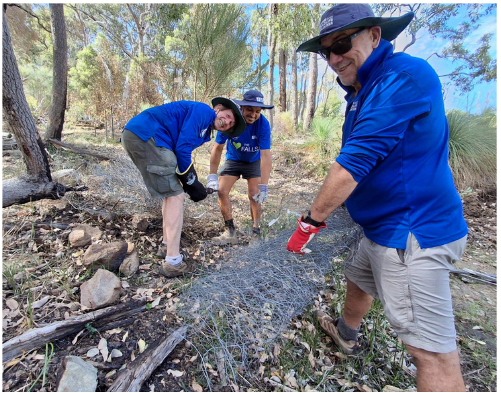
Mark, Jarrad and Paul removing the damaged fencing in the Erosion Gully.
