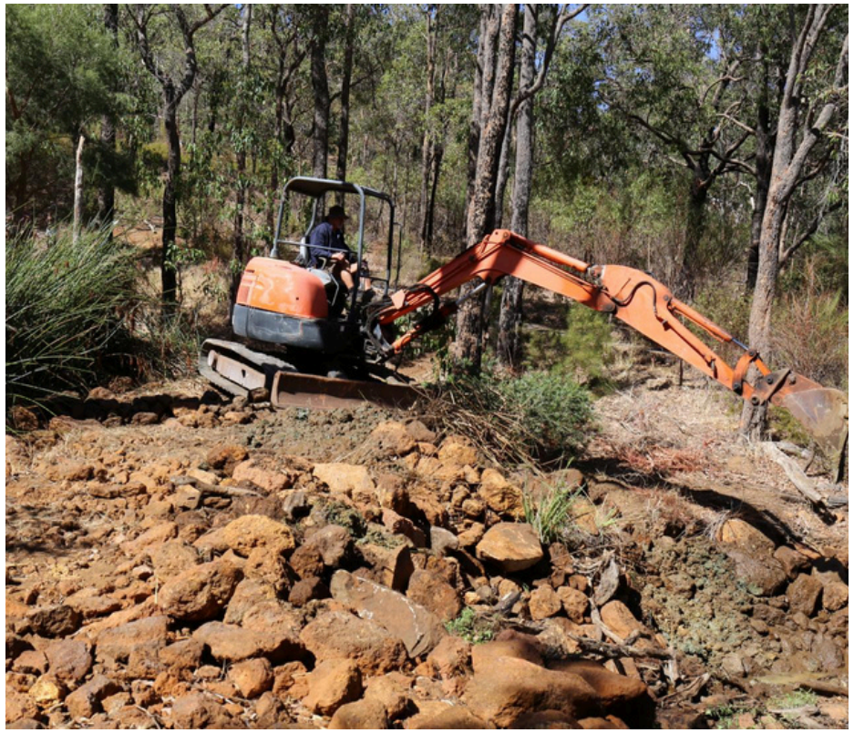
Our flow dams need regular structural maintenance.
