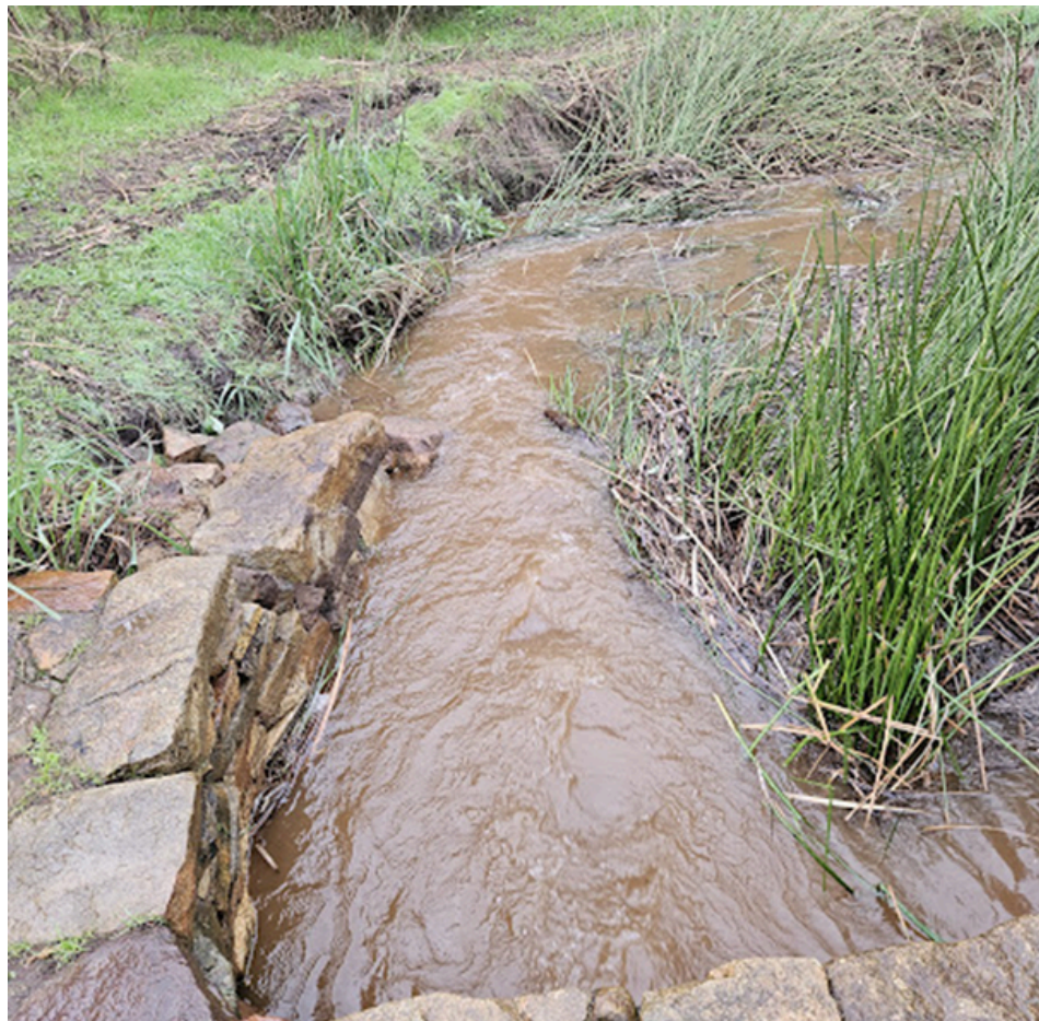
The waterflow from Guys Crossing after torrential rain a few days later - more rocks needed.
